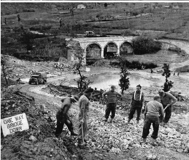
LEFT: A PARTY OF NEW ZEALAND ENGINEERS REPAIR A DEVIATION BY A DEMOLISHED BRIDGE.
