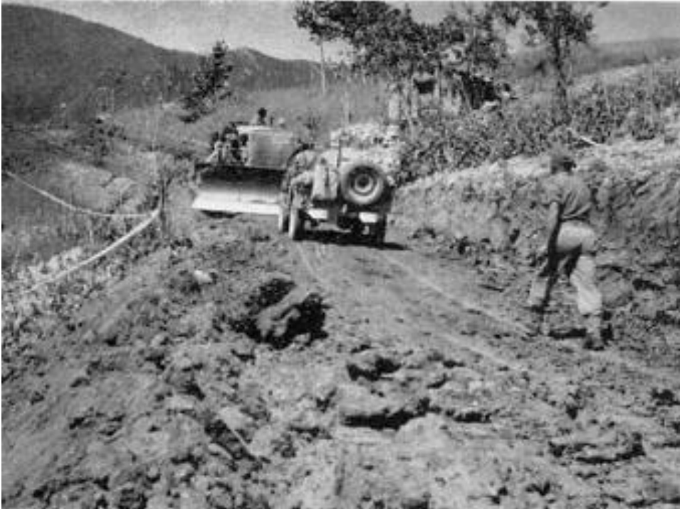
LEFT: DEVIATION ON THE ROAD TO AVEZZANO
